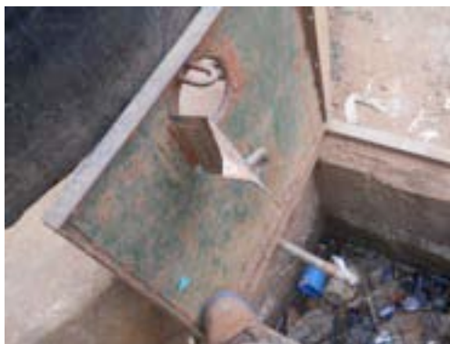
Current tap box at Bbanda R/C / Photo: EWB-NEU
