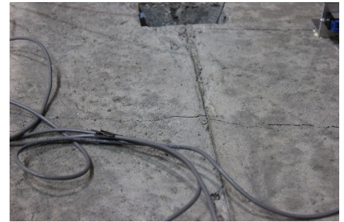
c) Longitudinal concrete cracks (parallel to the steel beam)
