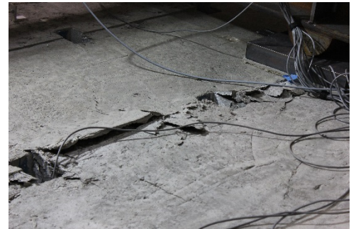
b) Concrete crushing at west interior loading point (plastic hinge region)
