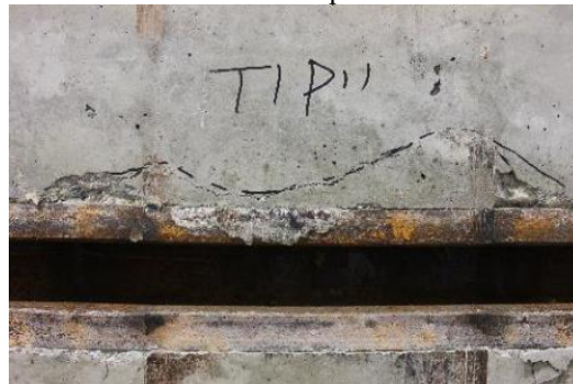
Cracking at the bottom surface of plank 11 in beam 1-M24-2C-RH Figure 5.40 Observations after deconstructing composite beams
