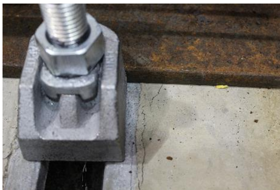
a) Crack at Clamp 3 at 0.02 in. slip
