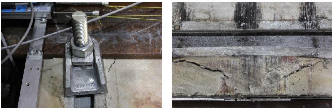
a) Concrete crack and rotation of Clamp 1 at 0.32 in. slip
